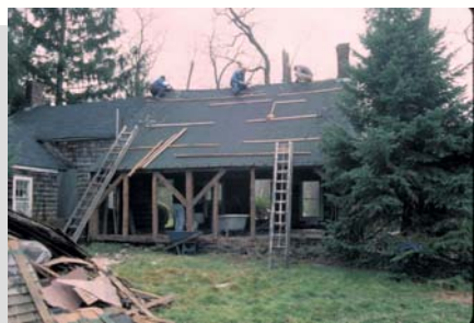
11-1-1993 The Samuel Hawkins House was constructed between circa 1720 and 1746 in two main sections. The timber frame is exposed and now the task is removing the layers of roofing.
